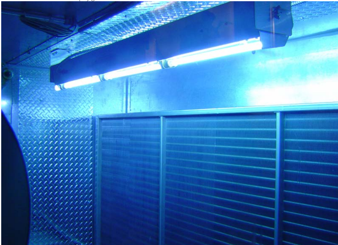
Figure 7: A UVGI system installed in front (upstream) of a cooling coil that sterilized the front face of the coil after two weeks of operation.
