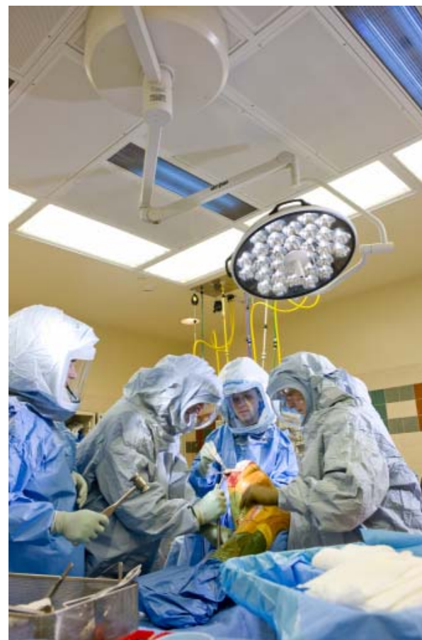
Overhead UVGI at St. Francis Hospital
