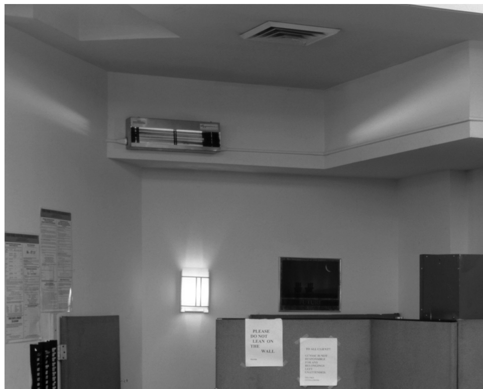
Louvered upper-air ultraviolet germicidal irradiation in Tuberculosis Ultraviolet Shelter Study New York City shelter. Photo: ©Randall Perry Photography.
